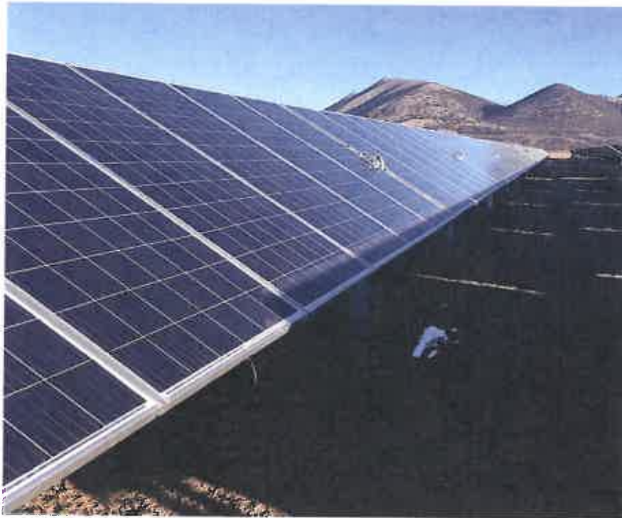
Figure A-3 – PV Module Array strings on single axis tracking racking (central OR)
