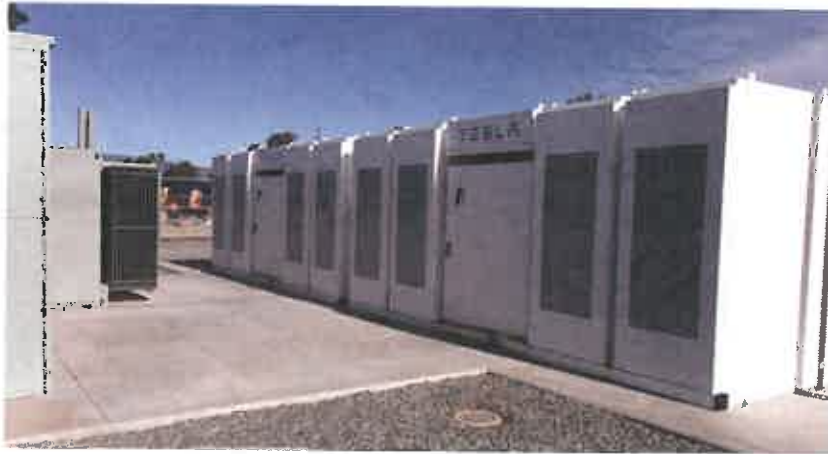
Figure A-5. Example inside substation, showing modular energy storage equipment, 34.5 kV transformers, breaker cabinets, and ancillary equipment on concrete mounted pads.
