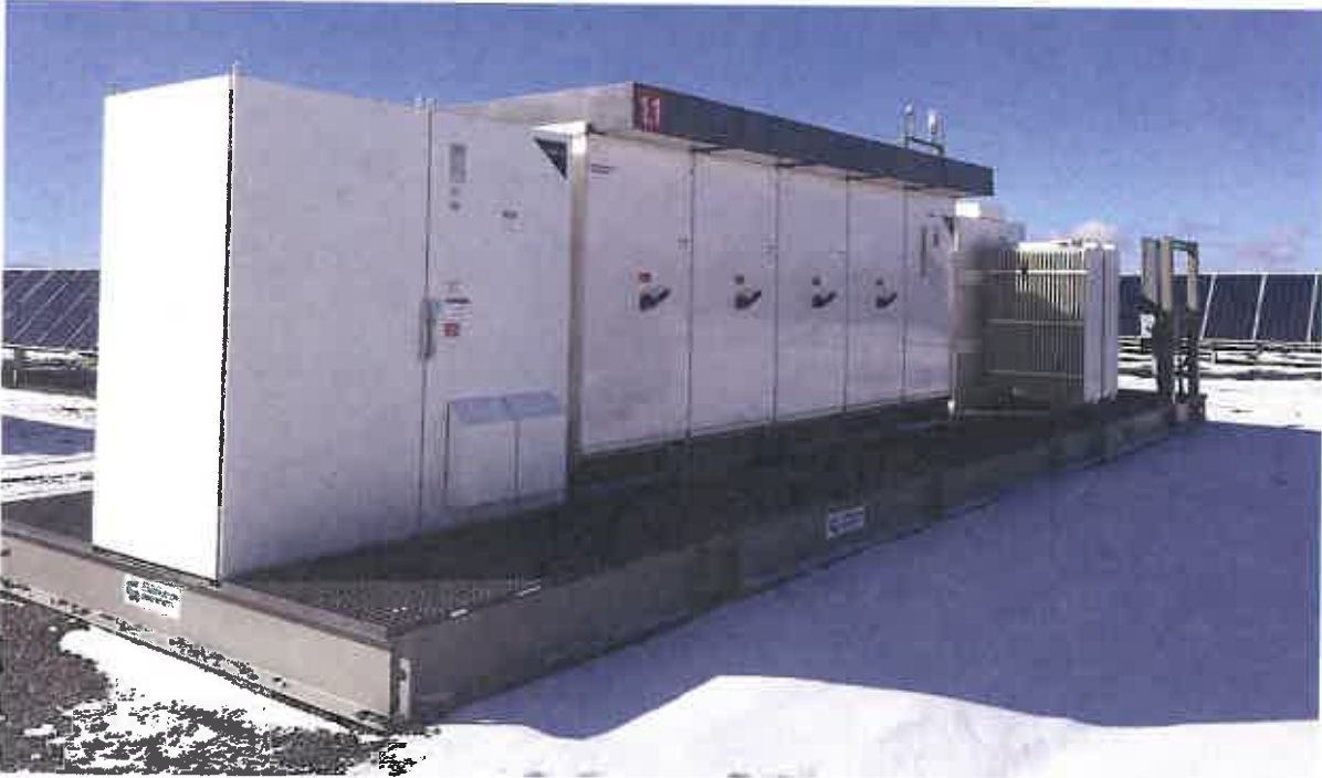
Figure A-4 Power Collection Station example in central Oregon.
