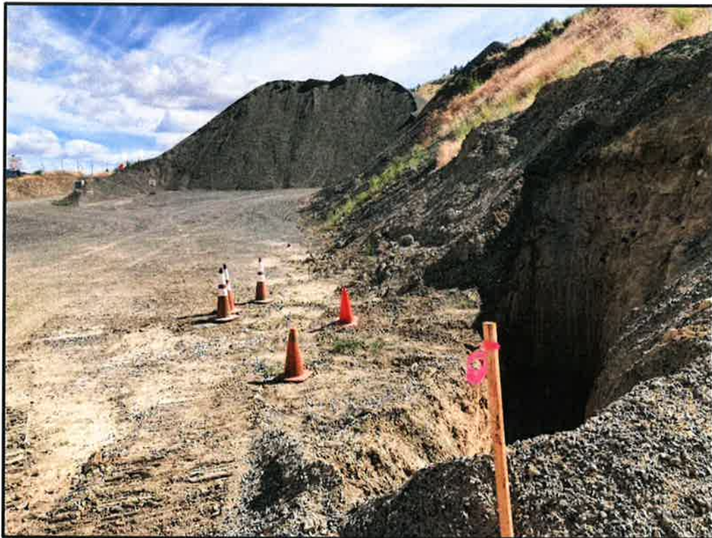
TP-01 at photo right. Note overburden silty sand overlying talus/scree unit. ¾" stockpile in background.
