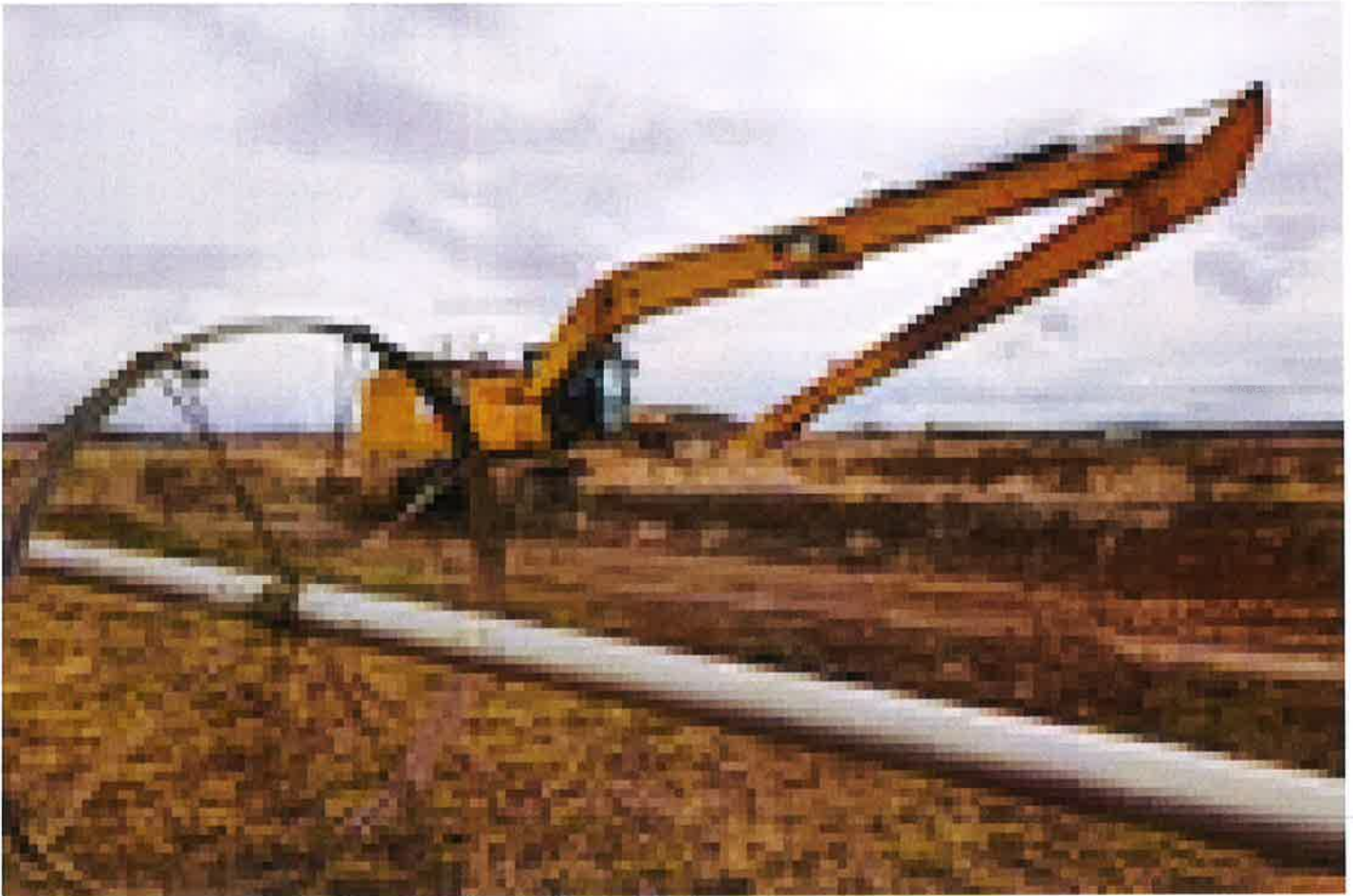
Heavy machinery mingles with irrigation equipment on the edge Knife River's Woodward pit in Crook County, Oregon. April 12, 2023 Emily Cureton Cook / OPB
